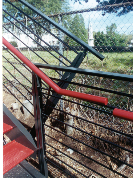
View of bent tube rail at bottom, left Top and bottom rail at landing, right
